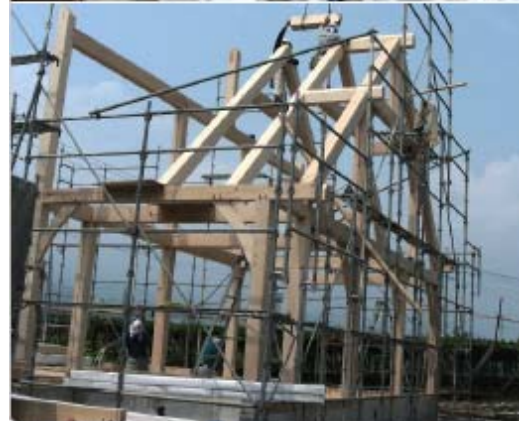
Timber-frame components & Building site in Kofu City, Yamanashi Prefecture – July 2007 The latest Timber-frame structure by the group – All Canada Tsuga Timbers
