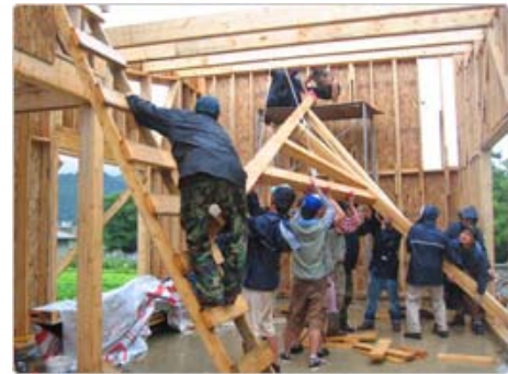
50 volunteers from 16 universities around Korea day and night constructing wood frame buildings worked round the clock.
