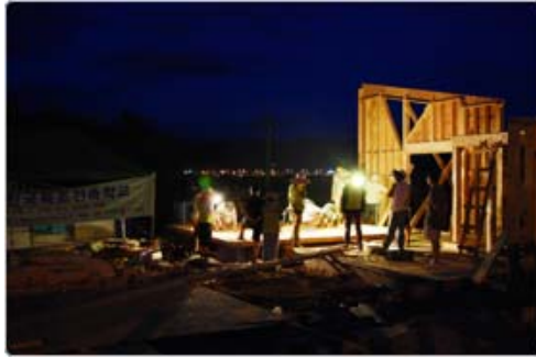
2,500 man-days were clocked from 27 June till 13 August to complete the wooden buildings from foundation to roof.
