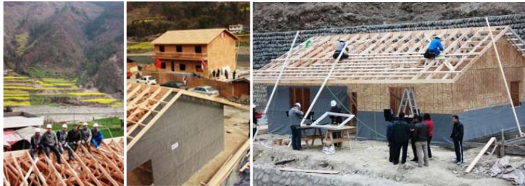
GUANZHUANG, QINGCHUAN: The 220 m 2 version (above) and the 80 m 2 version (bottom right) of Canada Wood's rural demonstration houses take shape. February 2009.
