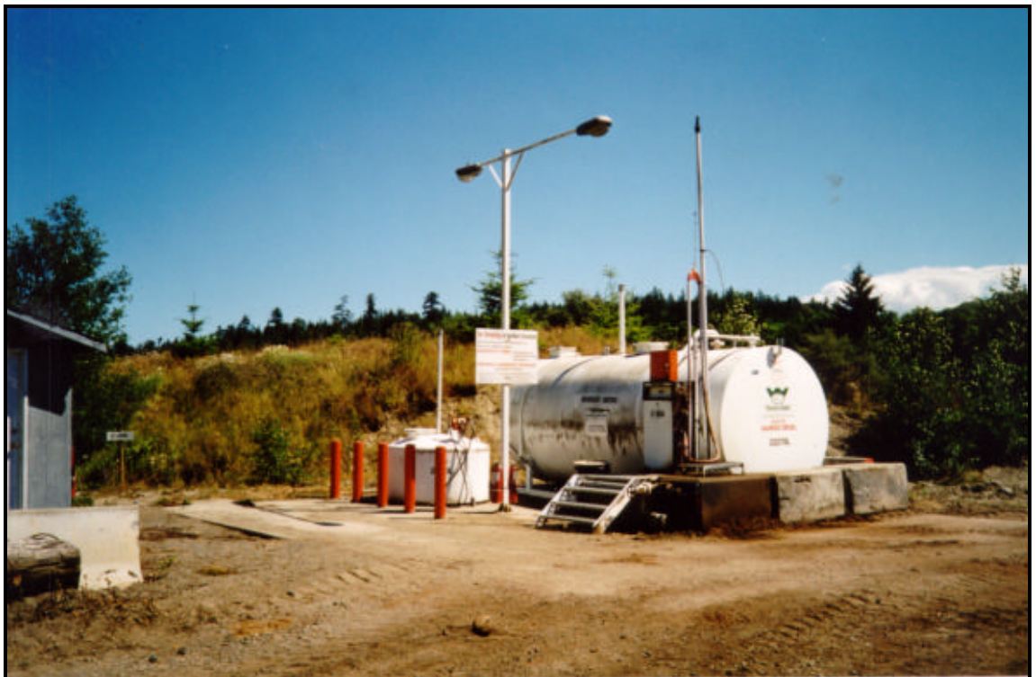
PHOTO6: Fueling station at dry landsort.
